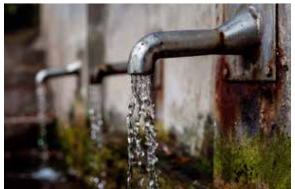
Domestic Water Supply
