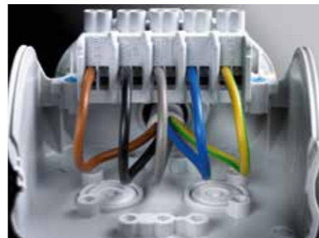
high-position terminals with more space for wiring
