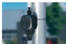
Power supply of a surveillance camera in public area
