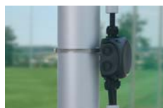
Lighting control of a sports field
