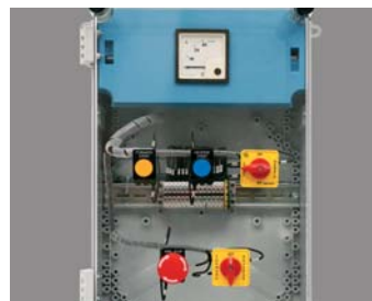
Waste water treatment plant to start / stop the pumps.
