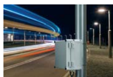
Control street lighting
