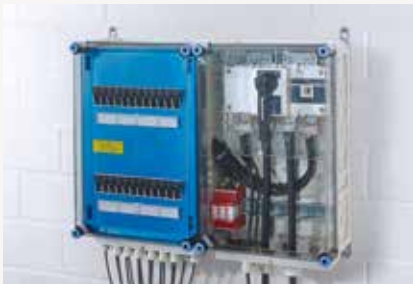
With surge arresters, string overload or blocking diodes if necessary
