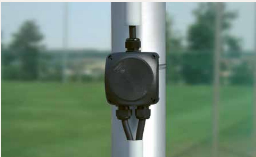
The KF series cable junction box was installed on a pole in a sports ground.
