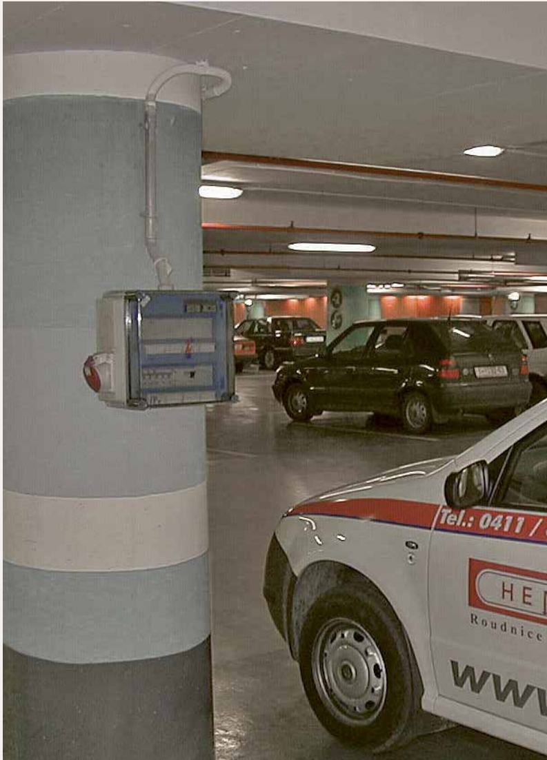
Mi distribution board in a shopping centre in the Czech Republic
