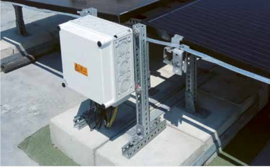
Numerous PV generator junction boxes are installed on the roof of a hotel.
