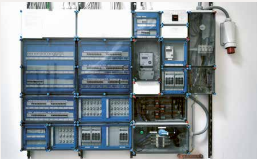
The Mi-switchgear provides safe energy supply in a fire station in Germany.
