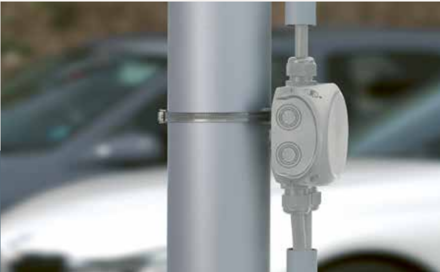
The HENSEL cable junction boxes with a mast fixing in a hotel car park
