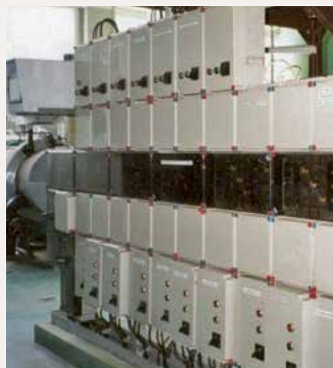
General power supply for keeping production processes up and running in a mine in combination with a generator.
