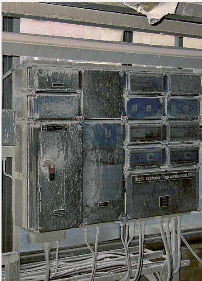
The distribution boards in a zinc mining company are exposed to extreme amounts of dust and dirt.
