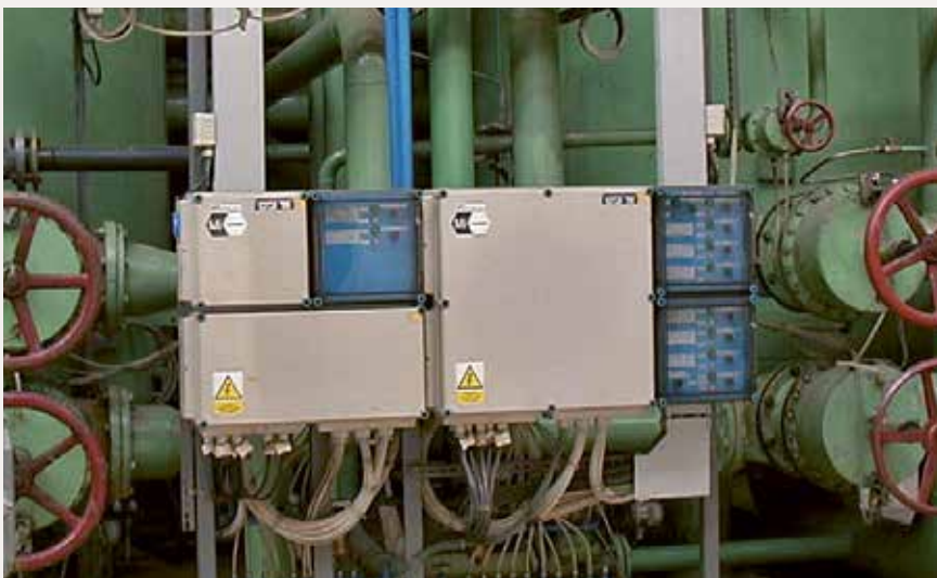
Mi distribution board in the chemical industry
