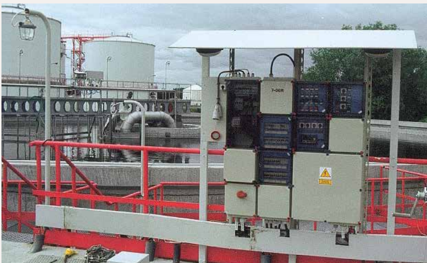
Water treatment and sewage plant in Danzig, Poland
