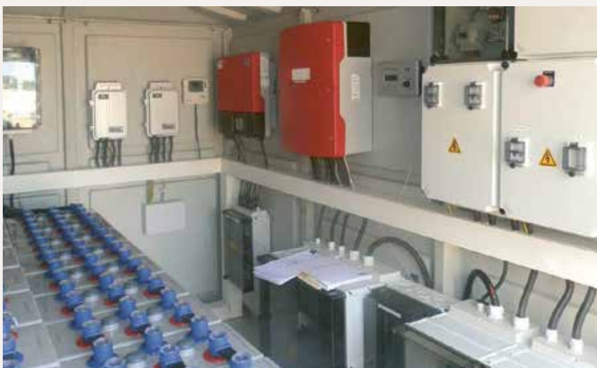
Electrification of railways with a power supply in the Congo
