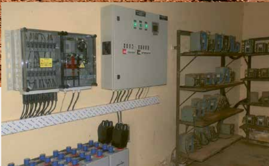
Electrification of a village in Liberia with PV generator junction boxes, PV power inverter collectors and battery distributors for protecting battery banks
