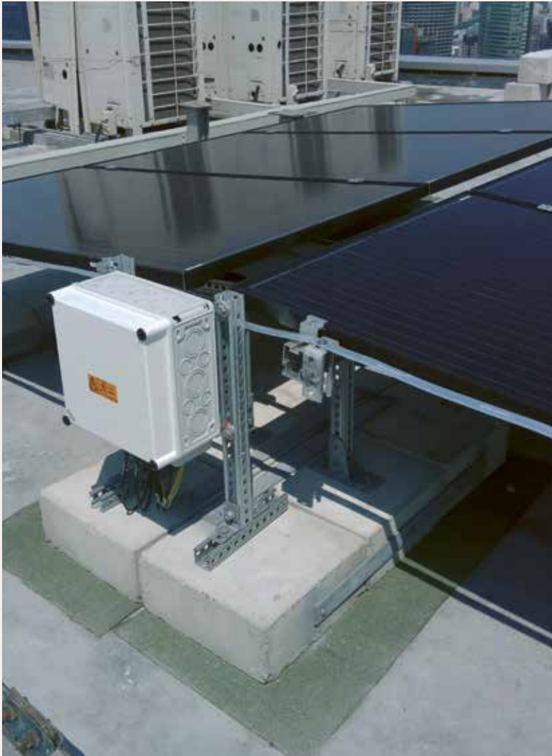
Numerous PV generator junction boxes are installed on the roof of the Marina Bay Sands Hotel.
