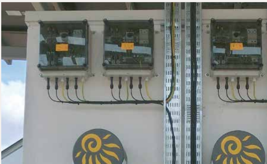
Numerous HENSEL PV generator junction boxes ensure a reliable distribution of generated PV electricity.
