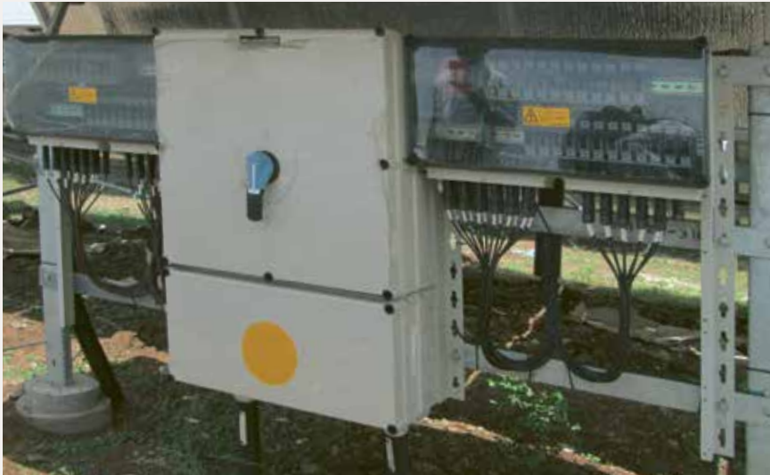
PV distribution boards before the expansion of a plant in Chennai, India.
