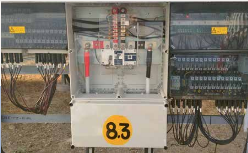
PV distribution boards after the expansion of a PV plant in Chennai, India.
