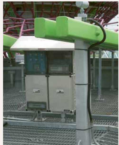
PV power inverter collectors are installed on the Supertrees in Singapore.
