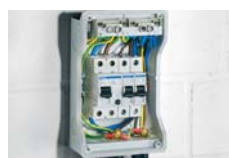
British Standard installation with earthed armoured cables
